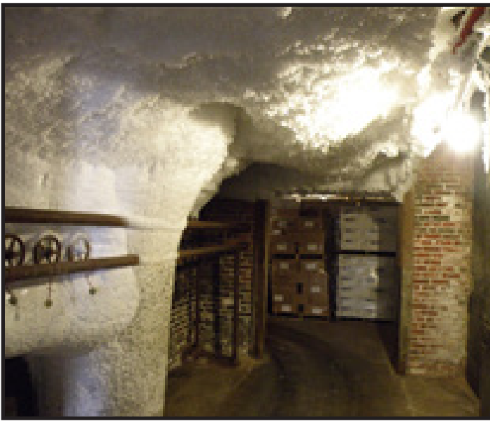
EPA inspection photo reveals dangerous ice buildup on ammonia piping and valves.
