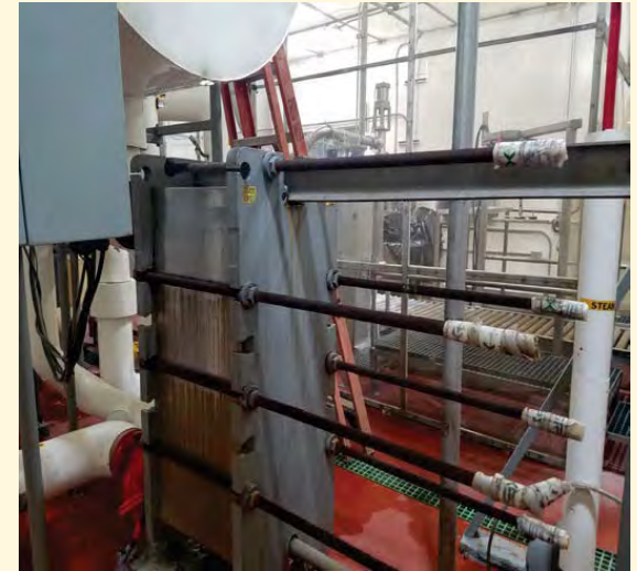
Secondary Refrigerant Cooling
