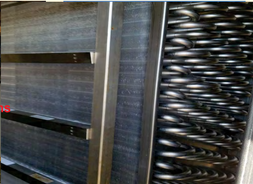
Air Handling Unit
