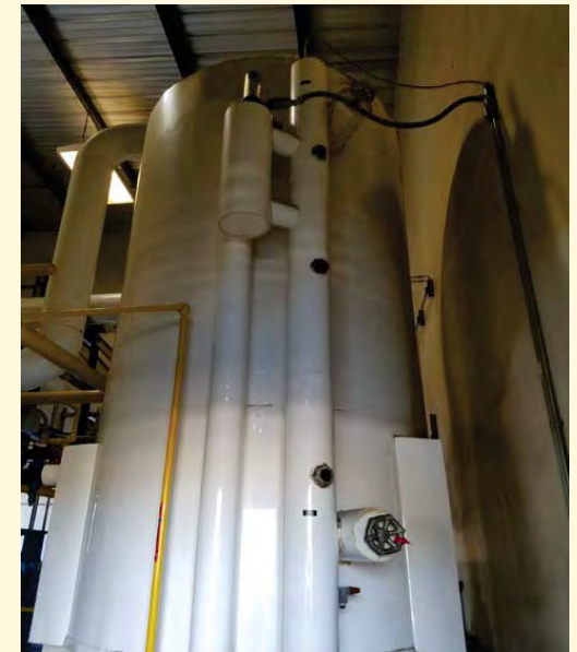
High Level Float
